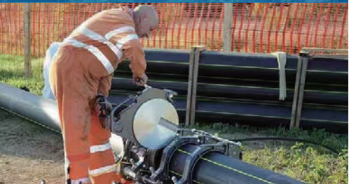
燃气管 Gas supply pipe
